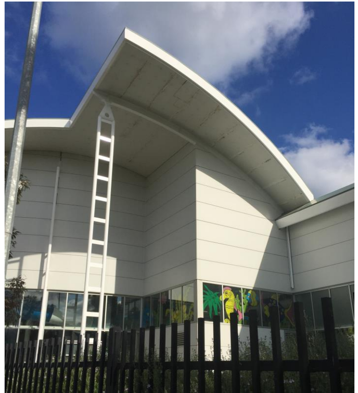
Damaged Eave linings
